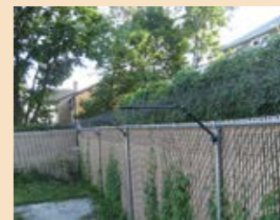
Conversion system on a Chain Link fence using U-Bolts to secure the arm mounting plate to the round posts.
